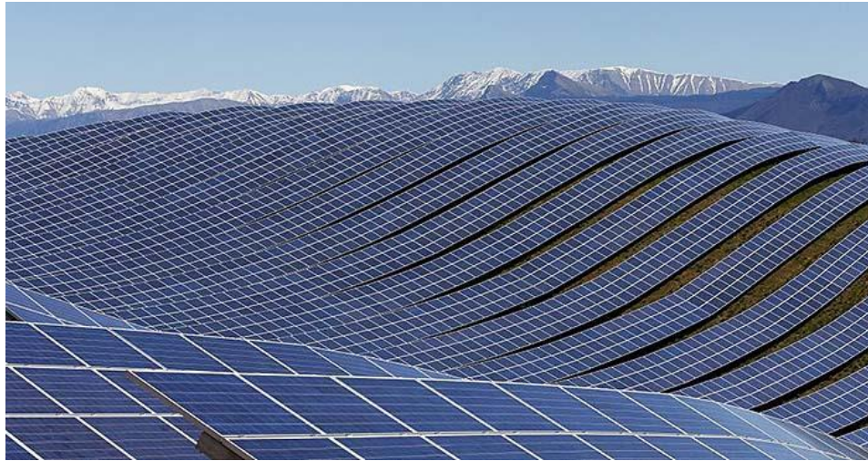
Fig. 2-2: Polycrystalline solar PV farm [2]
