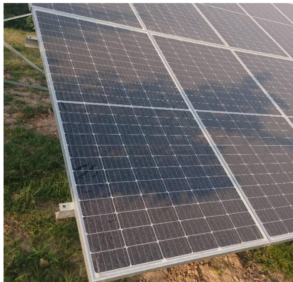
Fig. 2-8: Dust accumulation on PV modules
