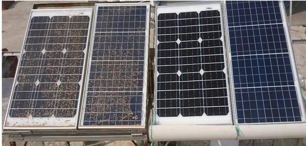
Fig. 3-4: Clean and dirty PV modules
