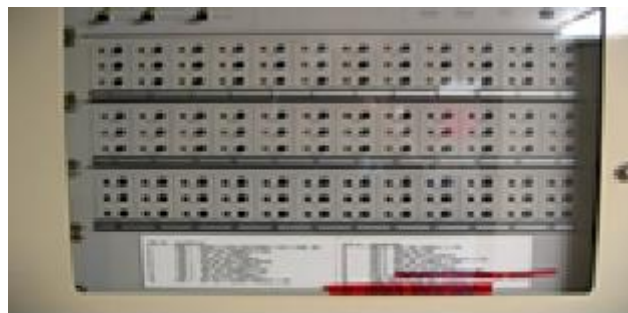
Figure 2.20: Fire indicator panel
