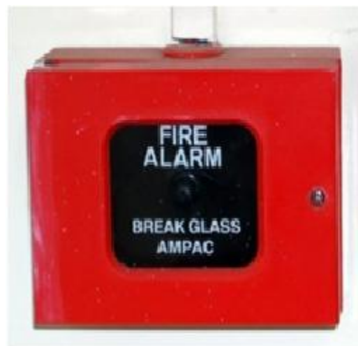
Figure 2.18: Fire Break Glass Alarm
