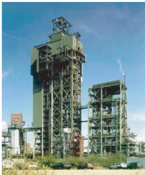
Figure 3.5 HTW plant in Berrenrath, Germany ©S.N. SIVANANDAM
