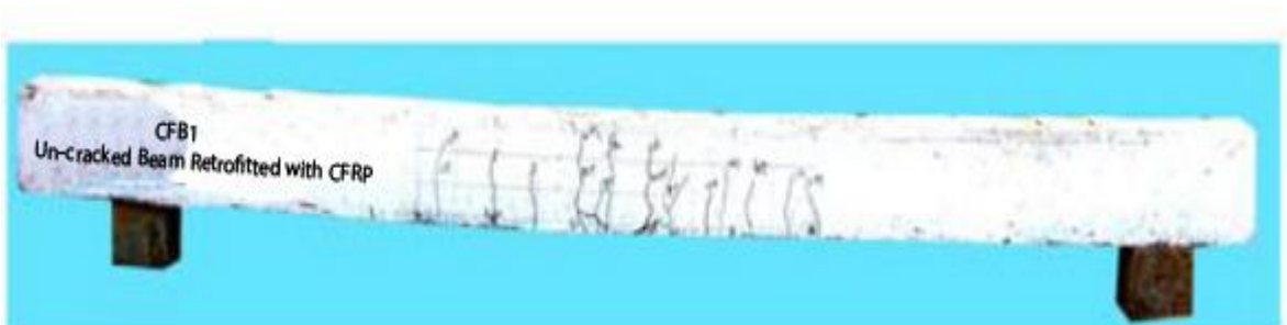
Figure 4-3: Cracking Pattern of Uncracked Beam
