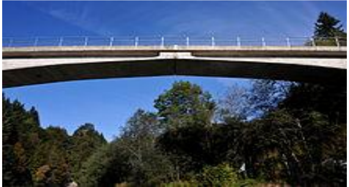
Figure 3.2 Rosssgraben bridge near Berne, Switzerland, showing the hinge at mid-span of this three-hinged arch
