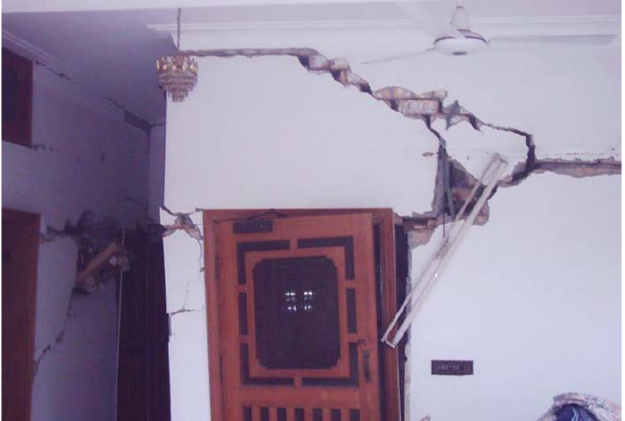
Figure 3.4: Failure of an unreinforced brick masonry wall in Muaffarabad, (EERI report, 2005)
