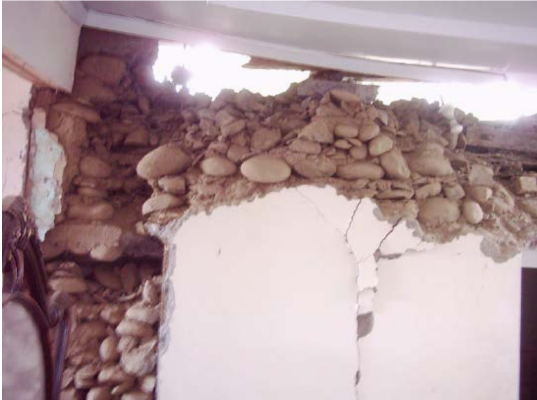
Figure 3.3: Failure of Stone Masonry walls in Kashmir 2005 earthquake, reproduced from EERI report, 2005.
