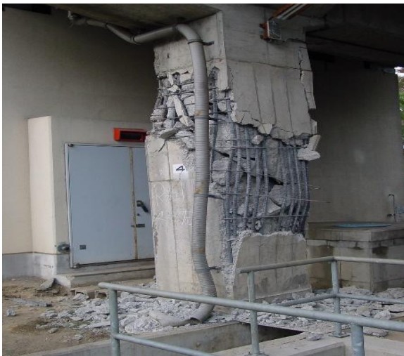
FIGURE 4-2 BUCKLING OF COLUMN
