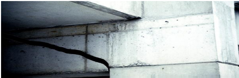
FIGURE 5-5 SHEAR CRACK IN BEAM
