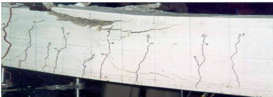
FIGURE 5-4 FLEXURE CRACKS IN BEAM
