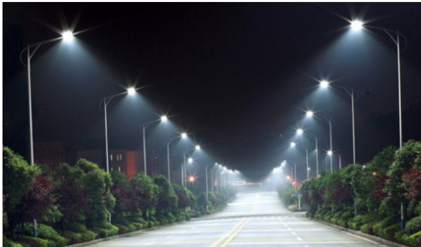
Figure 1-3: Conventional Street lights System
