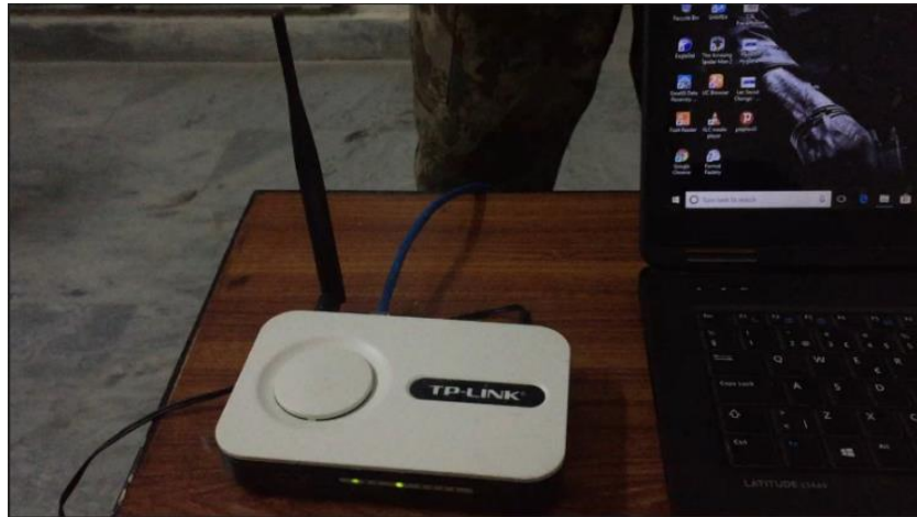
Figure 43: Router with its own Antenna
