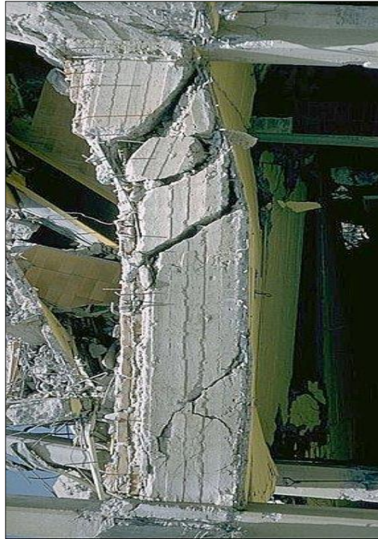
Figure 4. 7 Failure of a Column due to Shear Forces Generated in the Kashmir Earthquake
