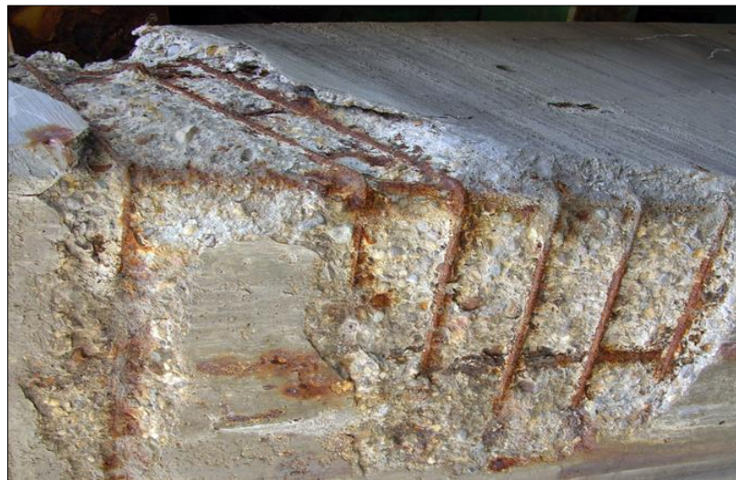
Figure 4. 6 Rebar Corrosion due to Inappropriate Cover
