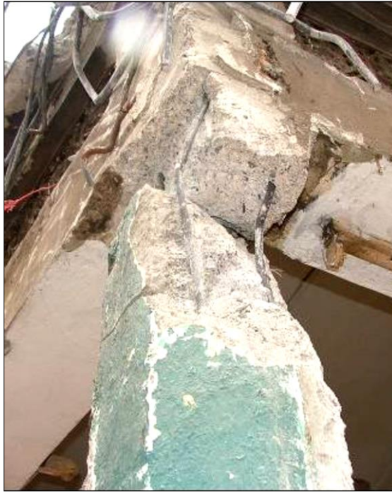
Figure 4. 15 Failure due to strong beam weak column arrangement (Kashmir, 2005)
