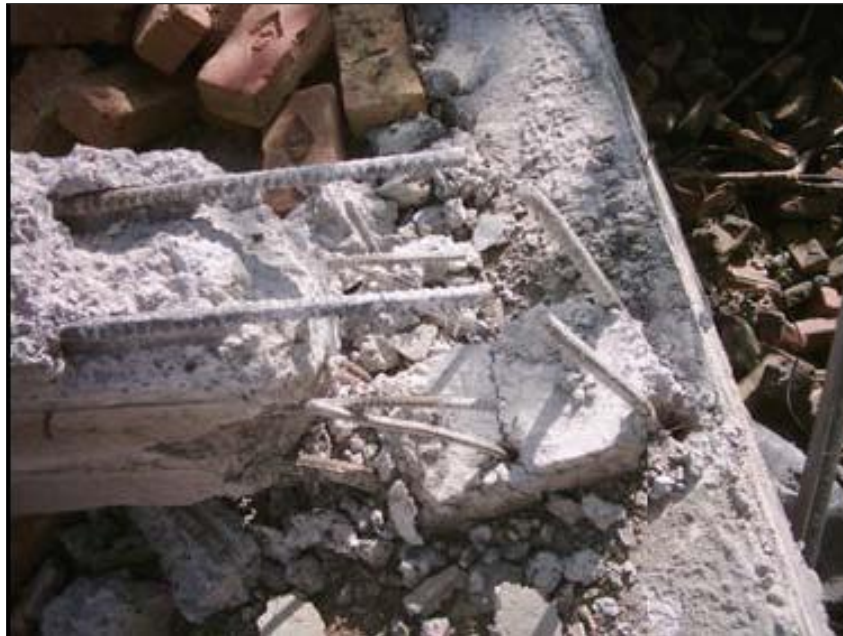
Figure 4. 12 Inadequate Development Length (Kashmir, 2005)
