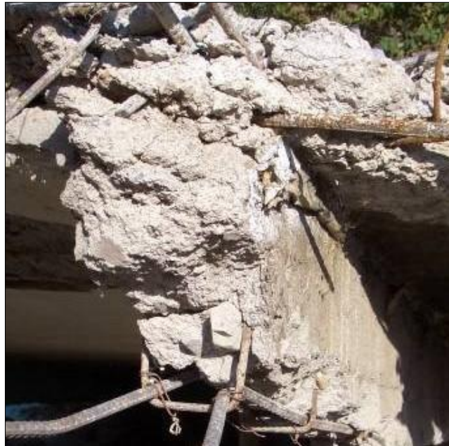
Figure 4. 11 Poor quality concrete subjected to seismic load (Kashmir, 2005)
