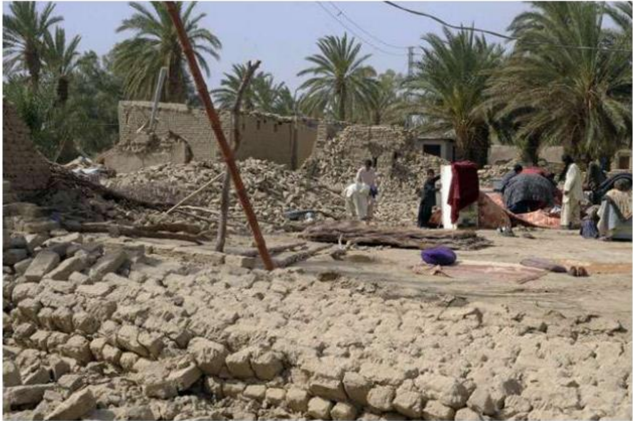
Figure 1.5 The Collapsed Weak Wall After the Earthquake (OCHA)
