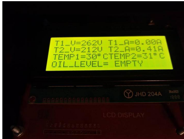
Figure 5. 2 Transformer readings on LCD
