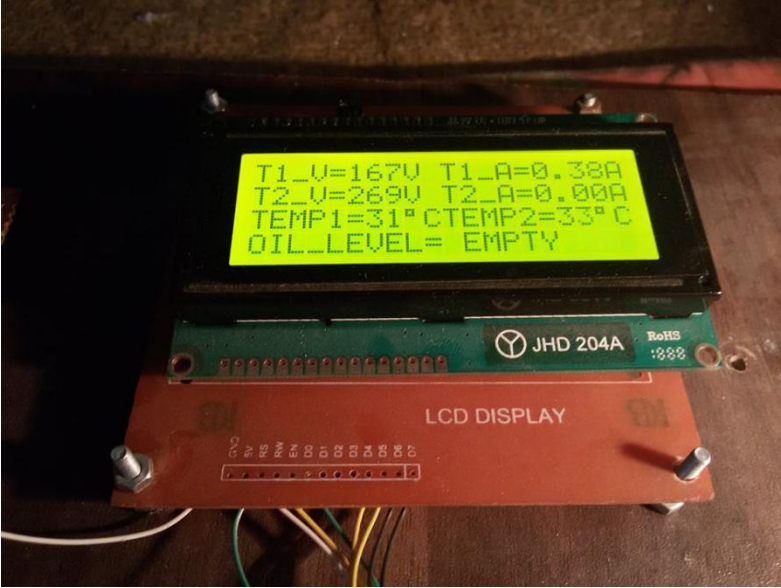
Figure 5. 4 Transformer 2 over volts condition on LCD
