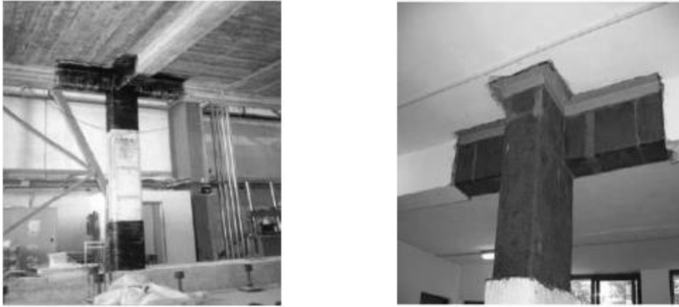
Figure 3. Retrofitting of RC beam-column joints with FRP (Tsionis et al. 2001 and Motavalli and Czaderski 2007).
